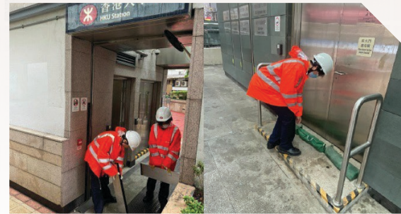
(Left) Operating colleagues installed flood boards at stations; (Right) Operating colleagues placed sandbags outside stations to prevent rainwater from entering
